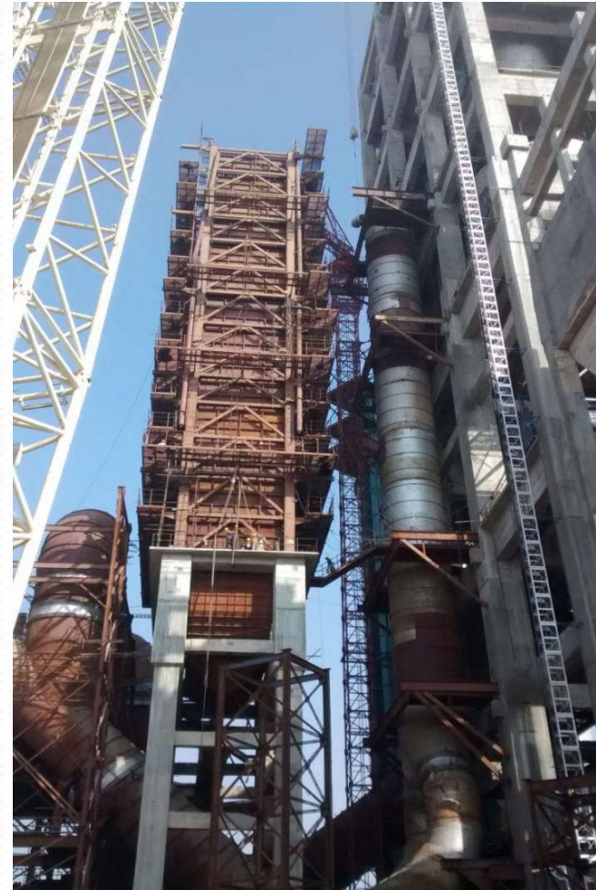
PH BOILER STRUCTURE, SHREE CEMENT, RAIPUR
