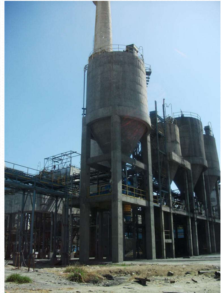
SILOS FOR ULTRATECH CEMENT
